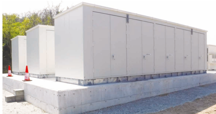
Grid storage battery systems
