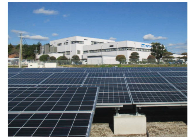
Solar power generation equipment (Oita Plant)
