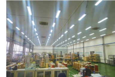
LED lighting in winding room
