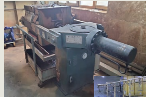
Waste water treatment unit
