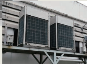
New outdoor air-conditioning unit
