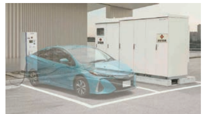
V2X emergency power system
