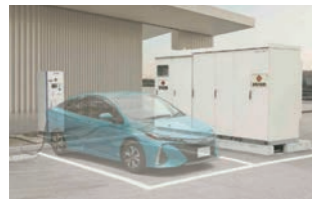
V2X emergency power system
