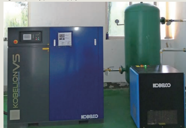
New air compressor
