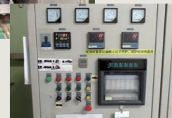
Drying oven control panel
