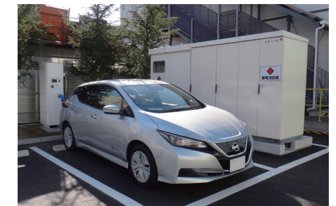
Pilot V2X System installed at Juso Business Office
