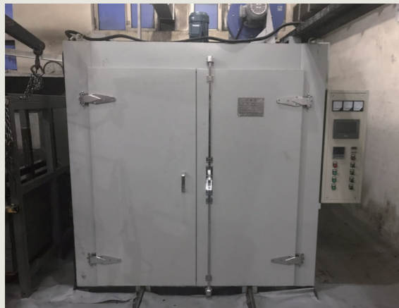
Newly installed drying oven
