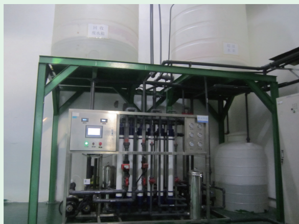
Wastewater recovery system
