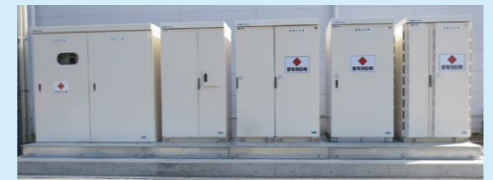
②-2 Storage battery system at the DAIHEN Technology Institute
