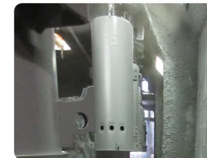
Coated transformer casing
