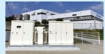
②-1 Solar power generation system at the DAIHEN Technology Institute
