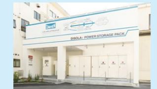
① Solar power generation + storage battery system at our head office
